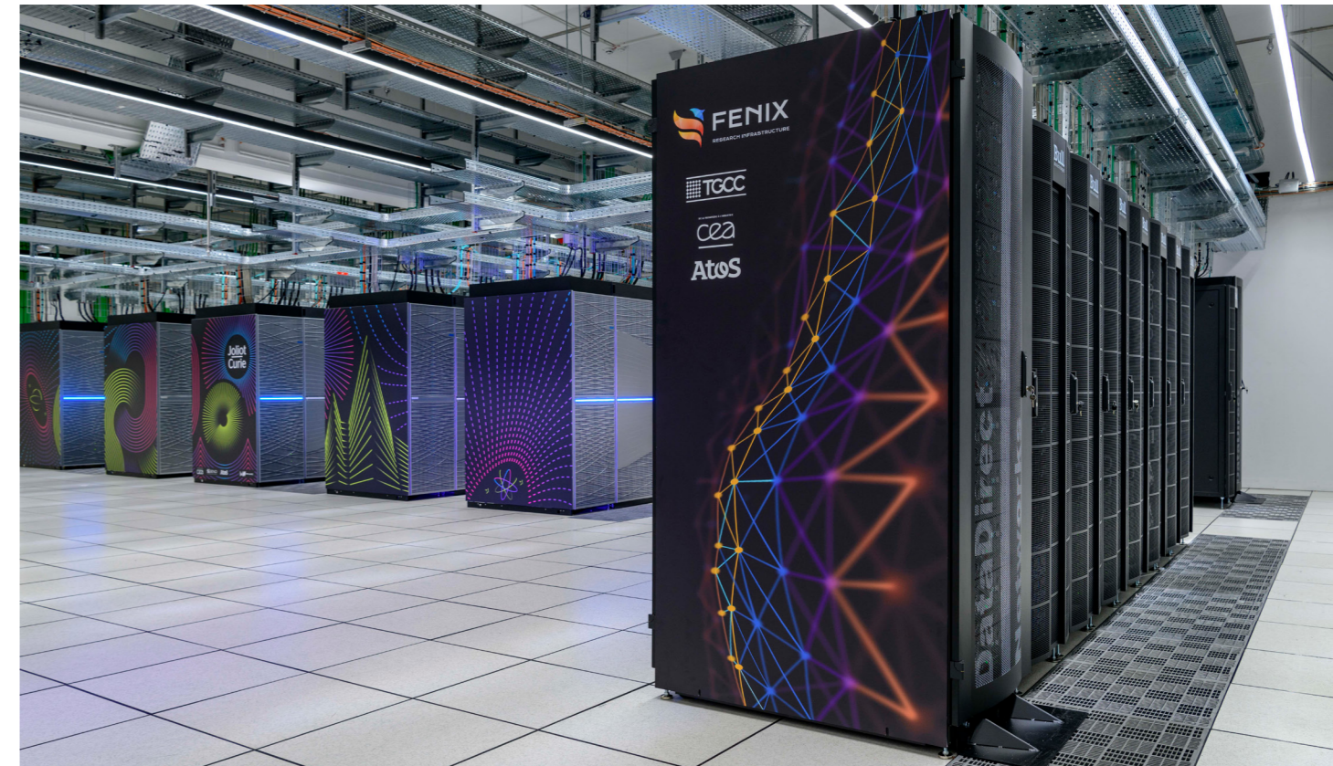
The TGCC computing centre of the French Alternative Energies and Atomic Energy Commission (CEA) is part of the Fenix infrastructure. © ICEI Consortium Partners
